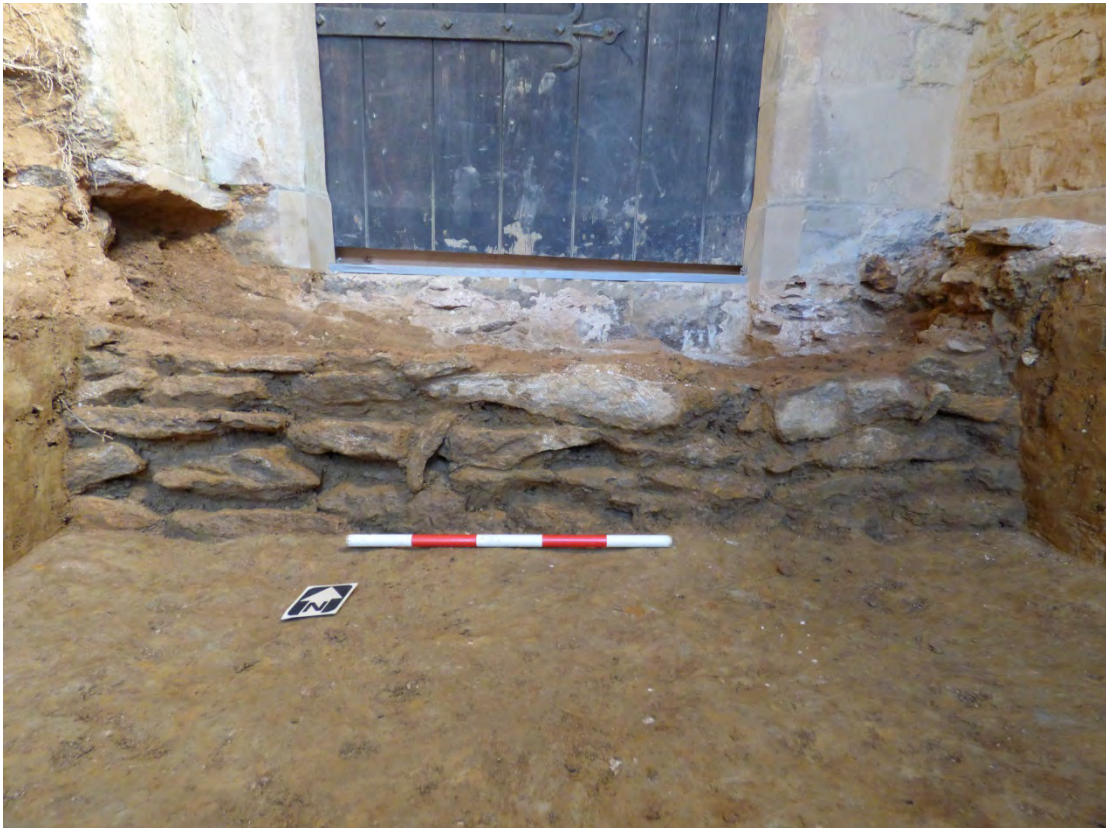
Nave wall foundations [45] cut through for the present south nave doorway. Level 1, soil horizon (65) in foreground, facing north Fig 7
