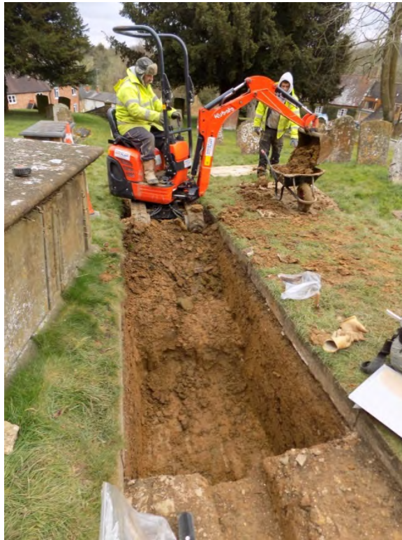
Service trench excavation along the churchyard path for the new soakaway. The transition point between the narrow and broad trenches, facing east Fig 14
