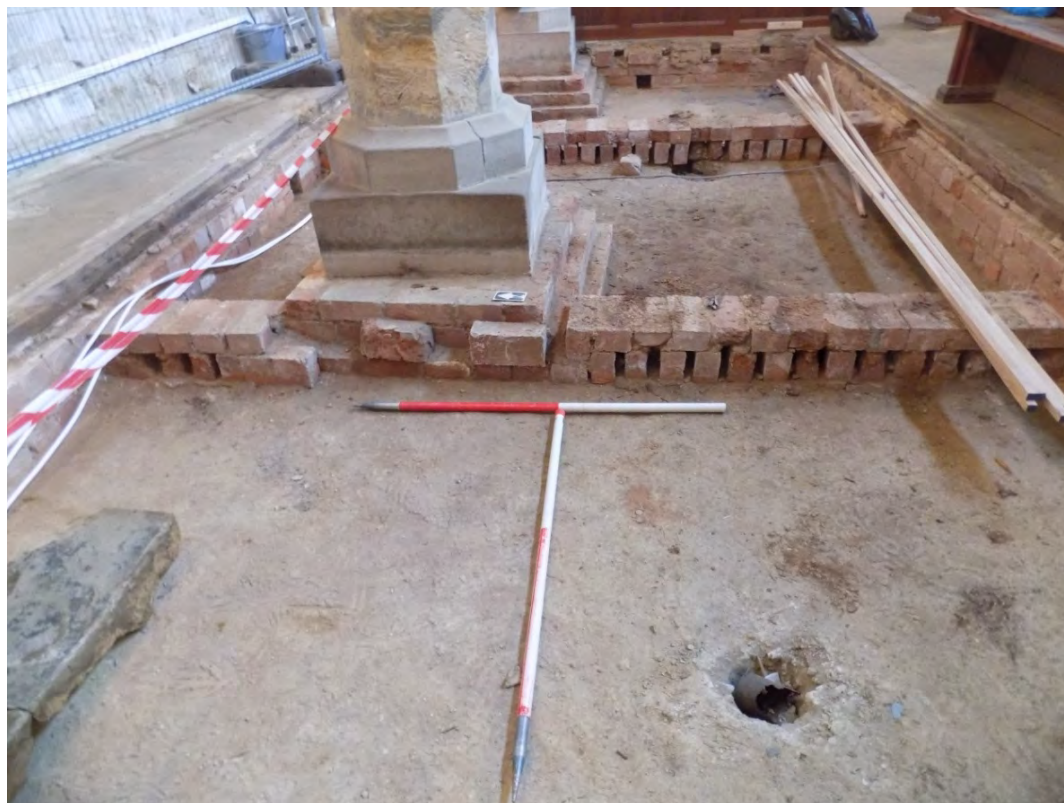
Bay 1, displaying the brick piers and the brick underpinning of the bases of the arch pier supports 1 and 2. Three scaffold post holes are also visible east-west cross the earthen floor (3), facing east Fig 18
