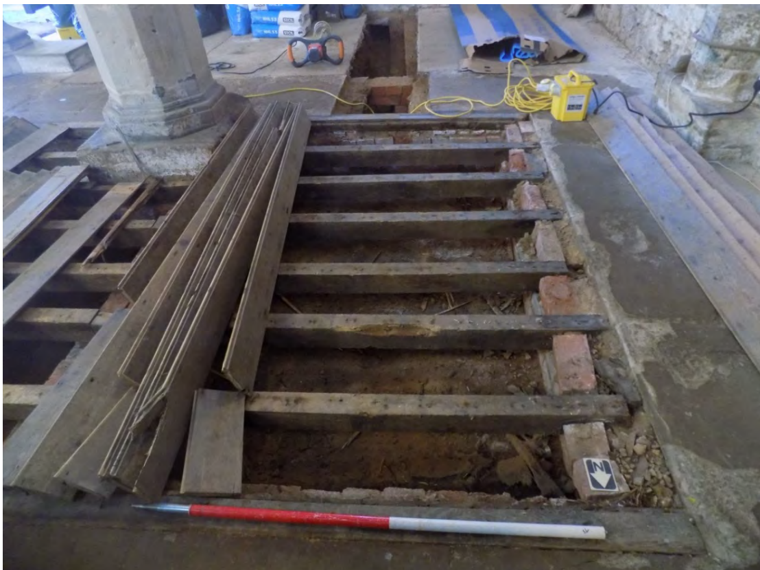
Bay 3, displaying floorboards (lifted) and wooden floor joists supported on the bay wall, facing south towards trench T1 (background) Fig 17
