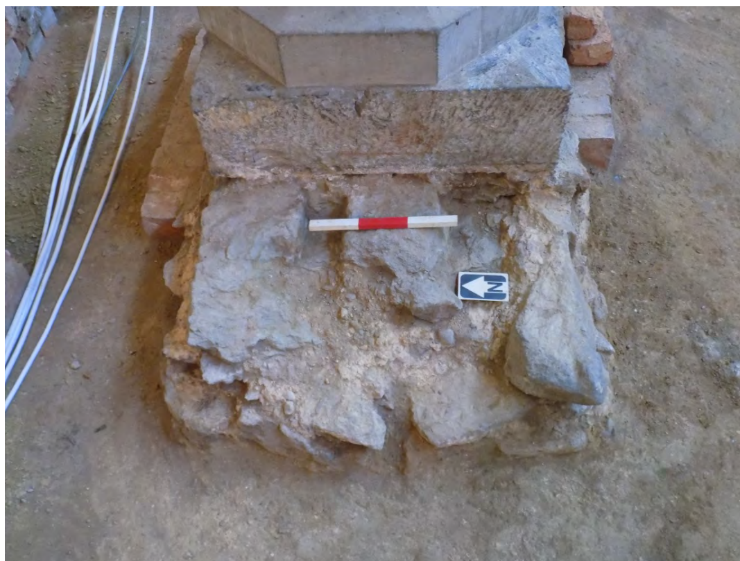
Bay 2 nave arch pier 4, with early stone and mortar foundations, facing east Fig 19
